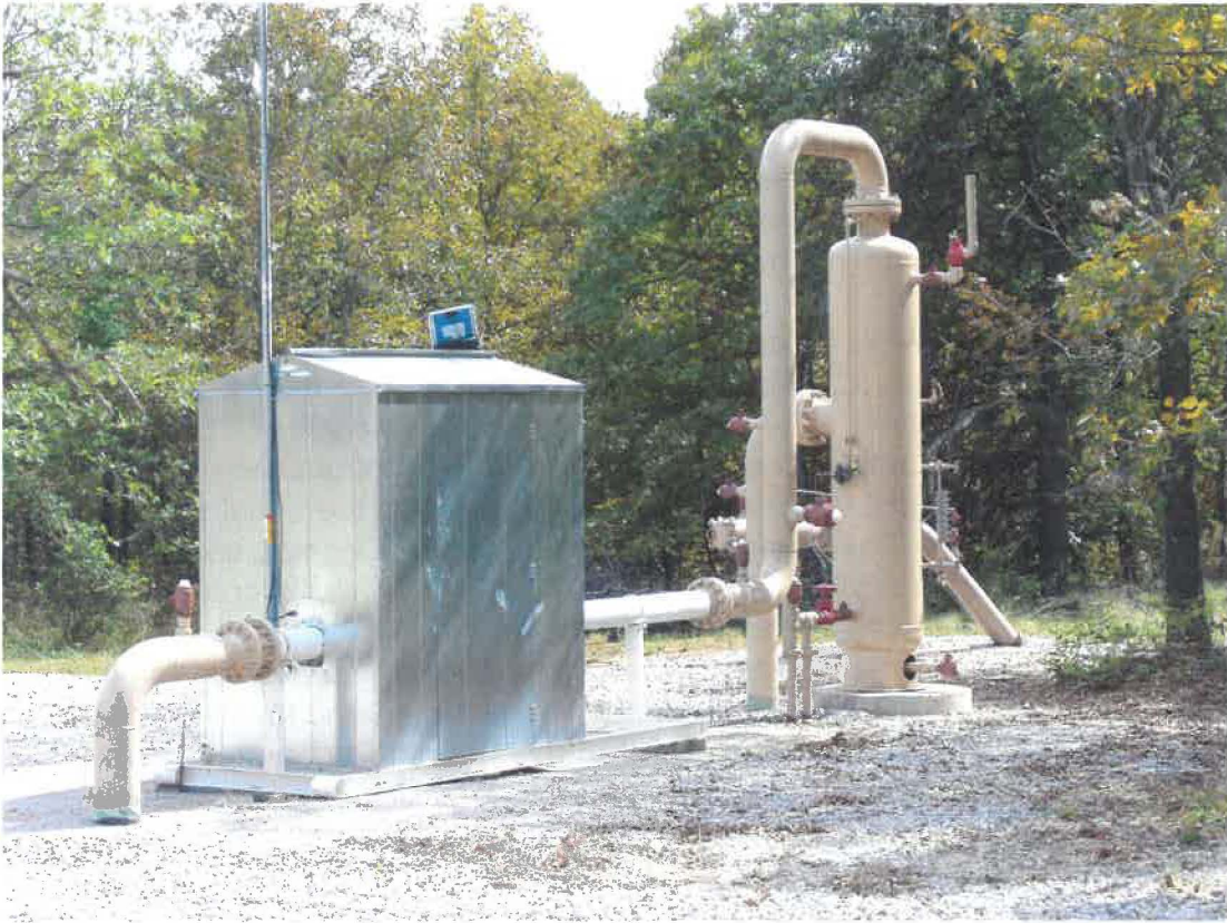
Inlet scrubber (on right) and inlet gas meter.
