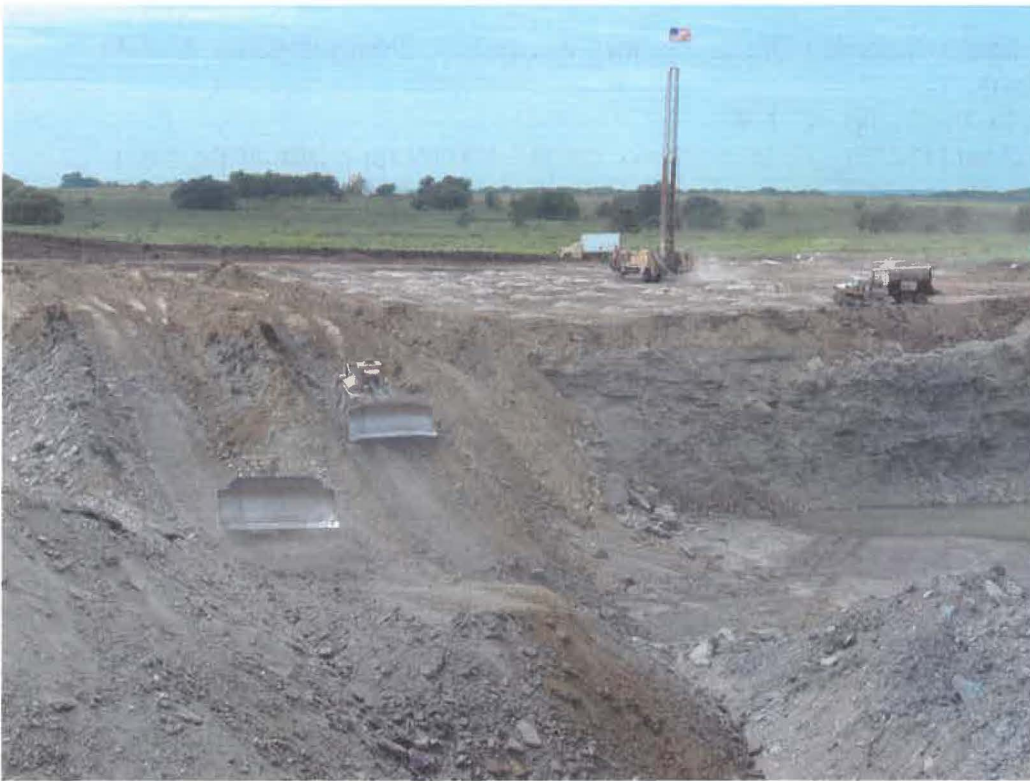
Caterpillar track-type tractors move overburden across pit. Drilling rig prepares holes to blast the overburden.
