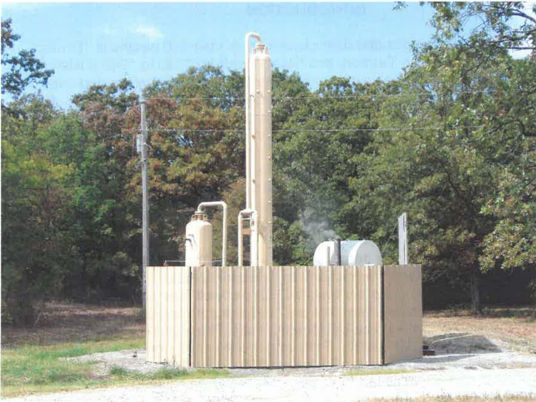
Dehydrator (removes moisture from gas prior to sales point)
