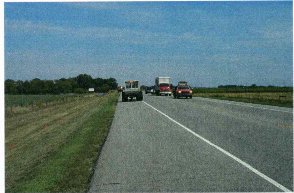
Fig A2. Vibrator along north road shoulder with KDOT pilot car managing traffic on U.S. 50.
