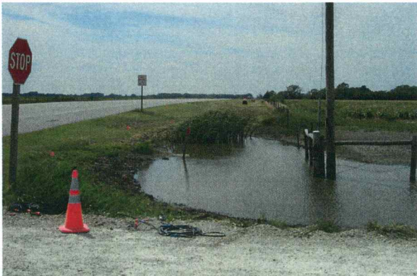
Fig A3. Sinkhole at the northwest corner of the intersection of Victory Road and U.S. 50 in Reno County.
