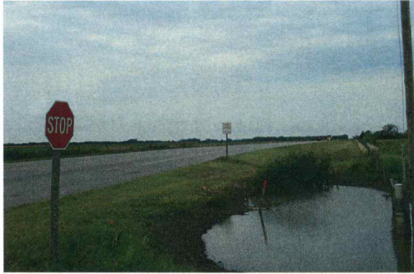
Fig A7. Looking generally west across sinkhole north of intersection of U.S. 50 and Victory Road.
