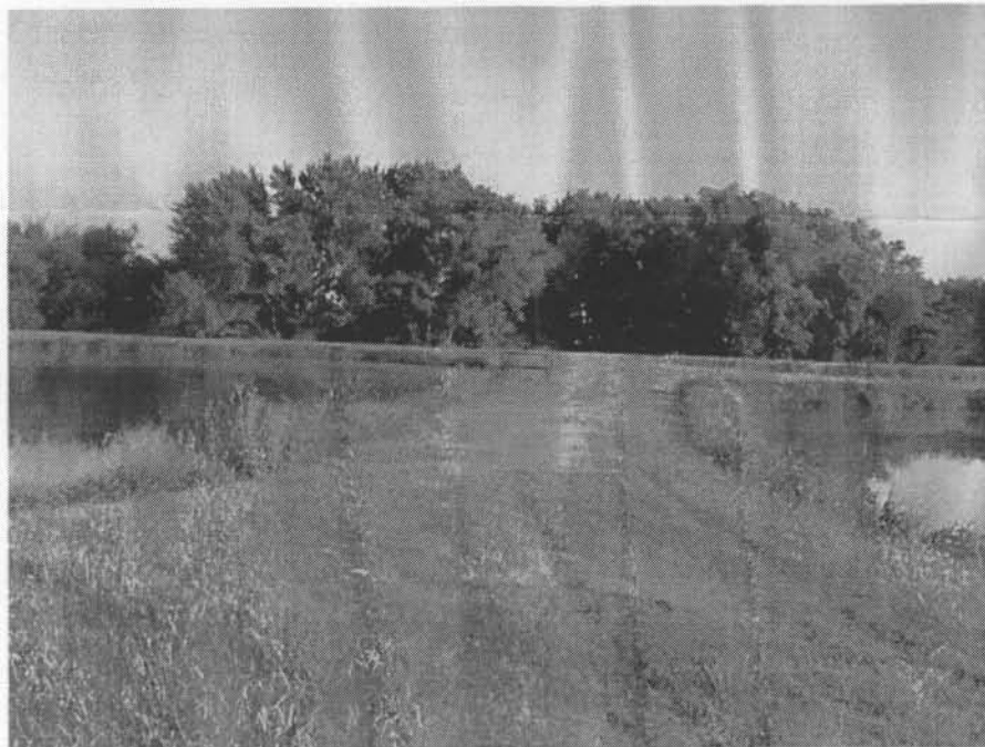
Eroded Embankments with Heavy Vegetation at Water Surface
