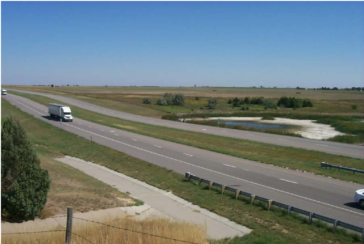
Figure 3. View of Crawford sinkhole from north approach overpass looking southeast, October 2003.
