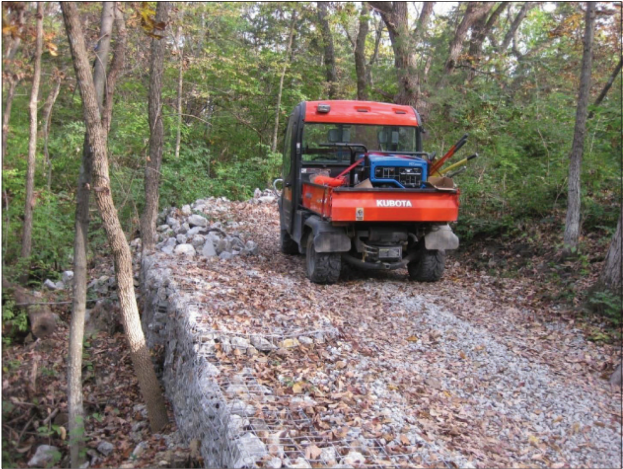
Figure 3. Rocks are hand placed in gabions, or wire cages (upper), to create a level double-wide trail in Kaw River State park (lower) (photos by Jeffrey Bender, KDWP).
