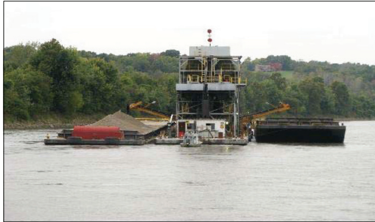
Figure 4. Stern view of a cutter-head dredge with a loaded barge on the left and an empty barge on the right (USACE, 2011).
