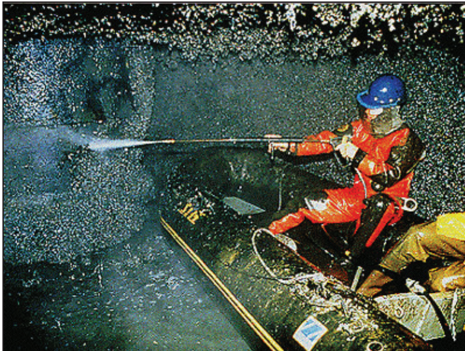
Figure 1. Water jetting being used to clean pump room at a condenser cooling unit of a power plant (photo courtesy of Aquatic Nuisance Species Information System [ANSIS]).
