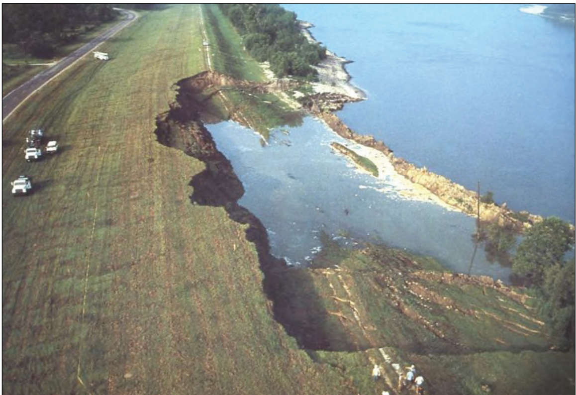
Figure 1. Example of a levee failure due to loss of foundation sediments removed by degradation (Shelley, 2011).
