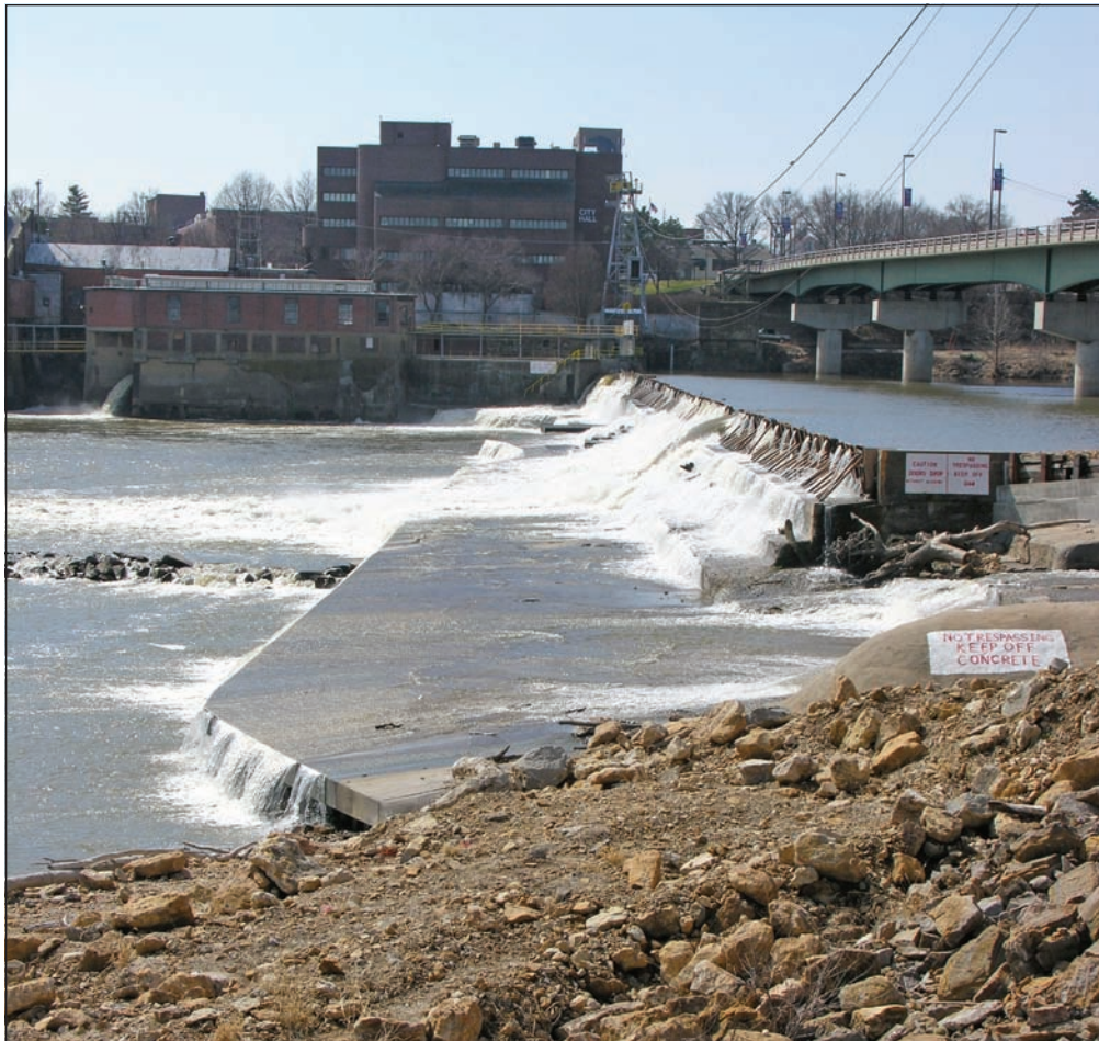
Figure 1. Bowersock Mills and Power Company (low building on river) and dam (photo by Cathy Evans).
