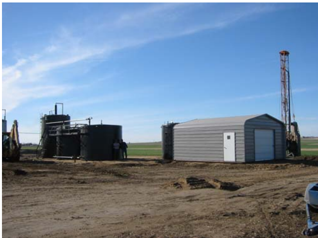
Figure 5. CO2 Injection plant near CO2 Project tank battery.
