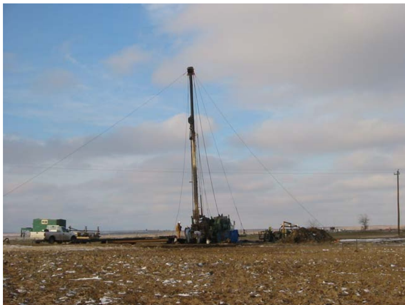
Figure 6. Workover rig on the CO2 Project #10 water injection containment well in early March 2003.
