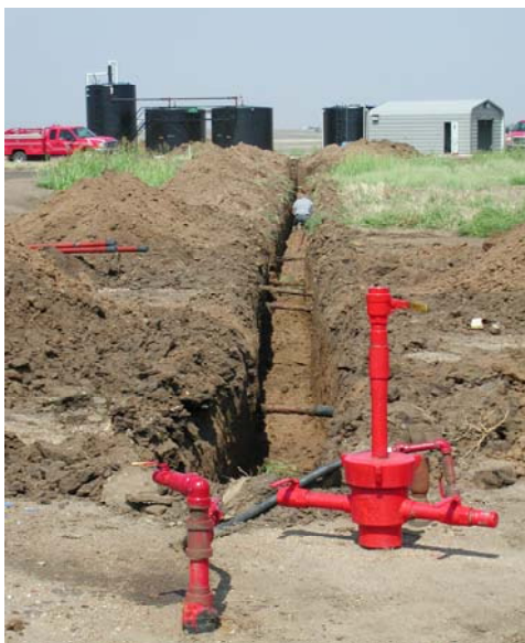
Figure 2. Laying fiberglass injection line from the water supply plant to the CO2#10 water injection containment well. View is looking to the northwest.
